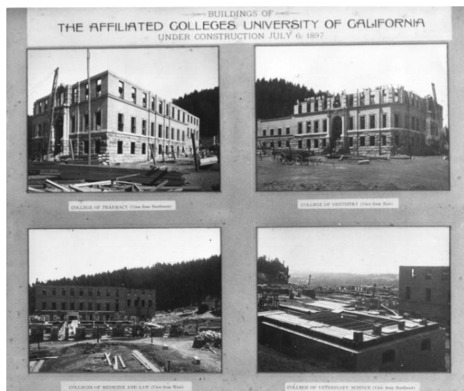
Figure 4. Buildings of the Affiliated Colleges, University of California under construction, July 6, 1897. “College of Veterinary Science” is in lower right. Source: Calisphere, UC San Francisco, Library, University Archives, https://calisphere.org/item/8b2c879f-56d4-4a53-b6f9-4b73c054a1cd/
